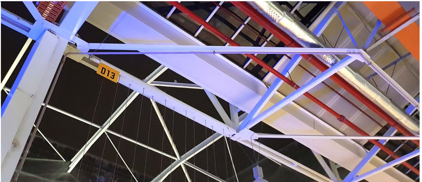
The irrigation pipes and control cables are housed in existing cable trays in the ceiling of the old factory building.
